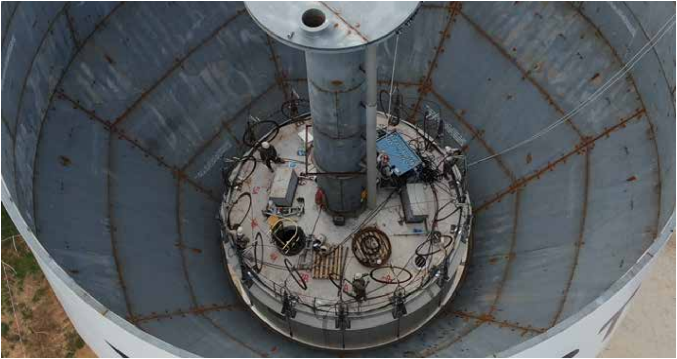
Workers help to raise and install a new water tower on Mary Drive near the Hurst Recreation Center.
